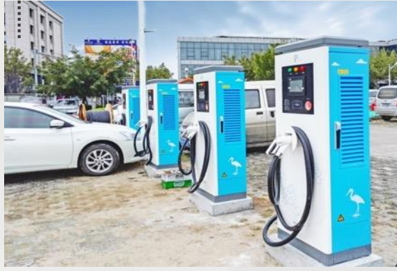
Xiamen Municipal Engineering Project, total charging power exceeding 3MW .
