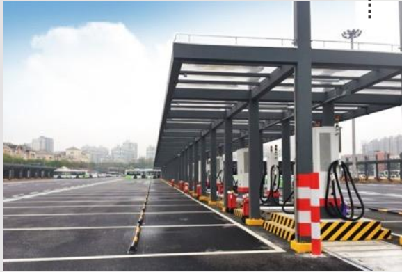
9.6MW charging station in Shanghai .
